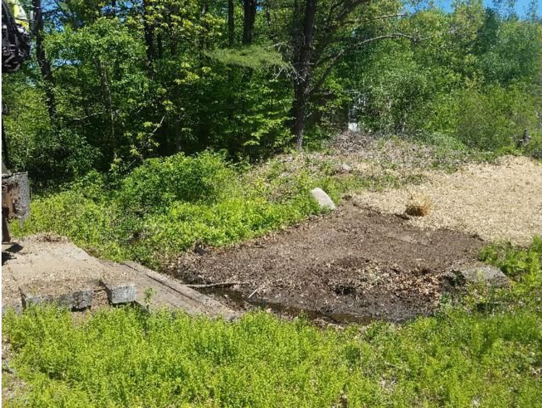
Fig 13: Removing timber mat bridge over stream NS8, next to Str. 102. Viewing north. (05-27-20).
