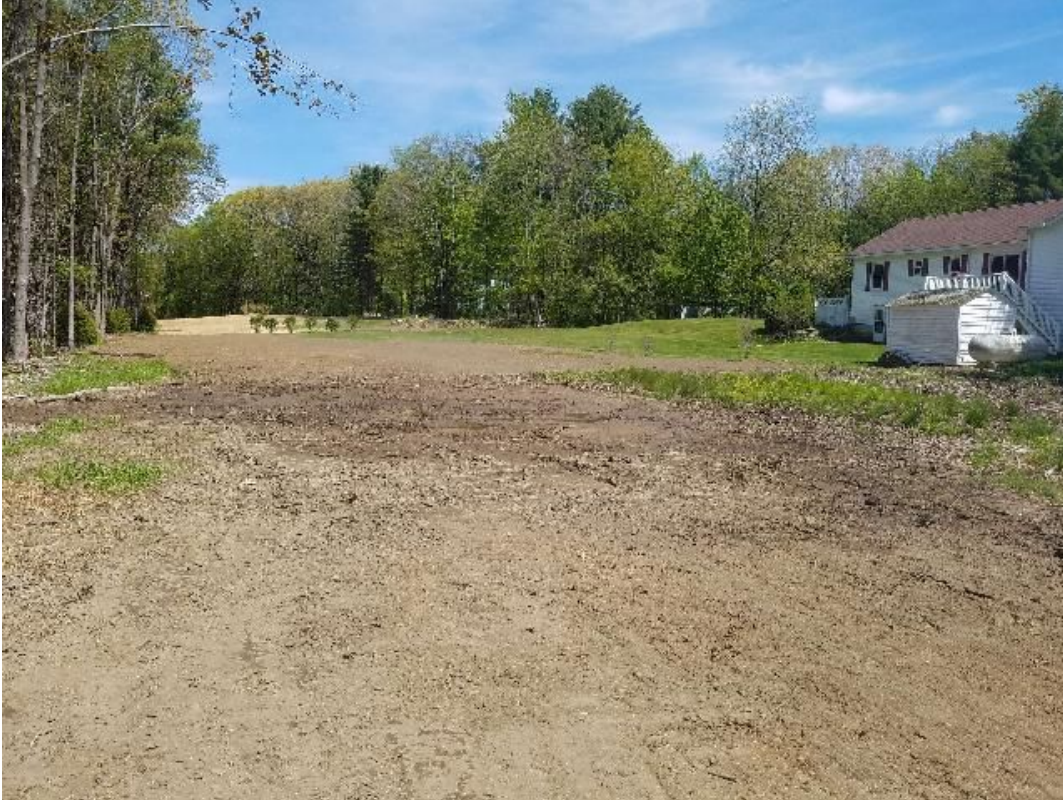
Fig 5: Restoration behind residential homes off of Hannah Lane. Wetland NW22. Viewing northeast. (05-21-20).
