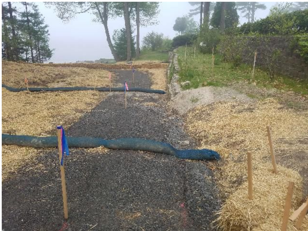
Fig 6: Area where additional rip rap swale will be installed on slope at Gundalow landing/east side of the Bay. Viewing southwest. (05-26-20).
